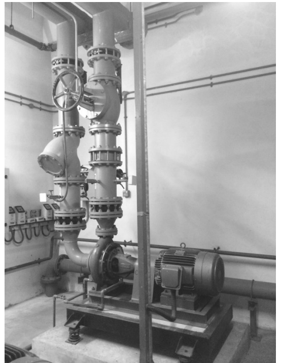
ပုံ ၆-၉ Condenser water pump pipe connection
