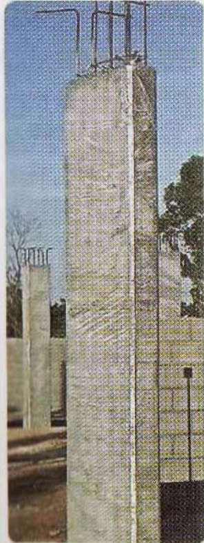
Plastic wrapped around a concrete column
