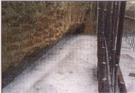
Undermined basement excavations in good soil remain intact for some time
