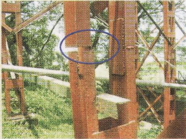
Faulty column connection
