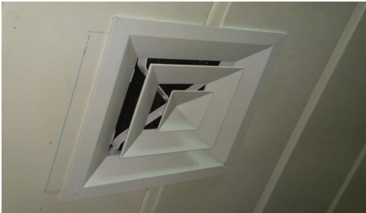
Figure 2. 4-way diffuser mounted at the ceiling
