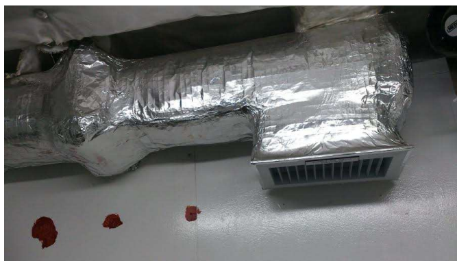
Figure 3d. Grille on the duct
