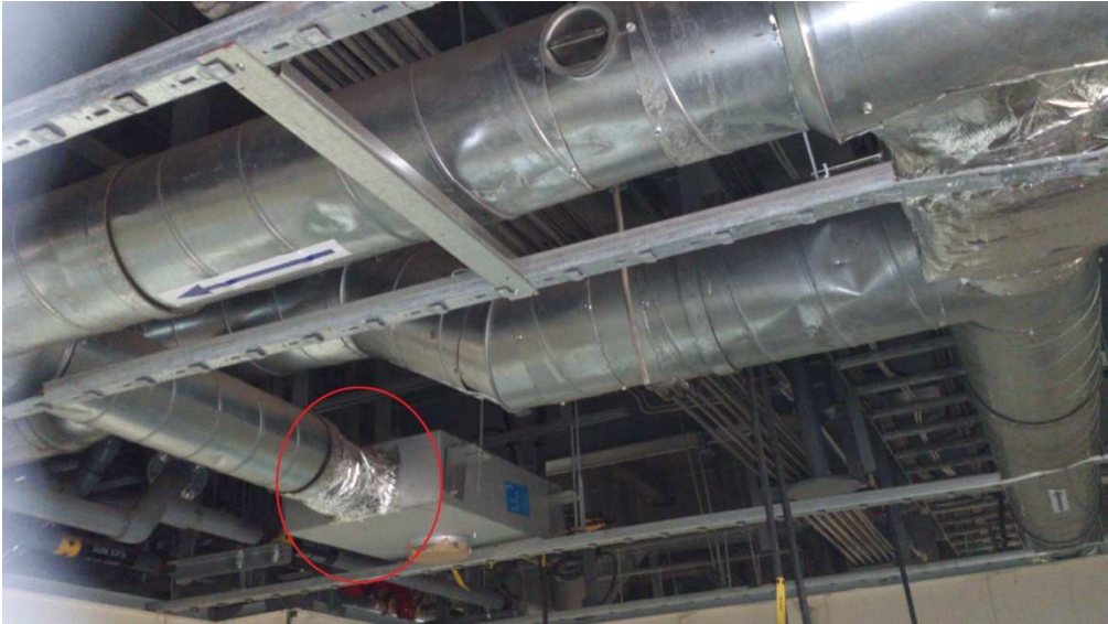
Figure 7. Flexible connected with cabin unit
